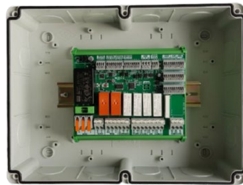
Power Base / Enclosure (Field installed on roof of cold room)
